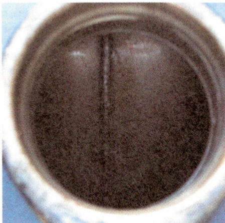
Gastank after: Properly applied; even coverage on all interior surfaces of the tank.
